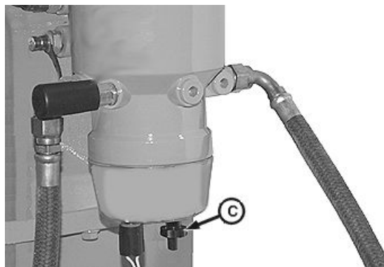
Draining Water Separator Bowl
